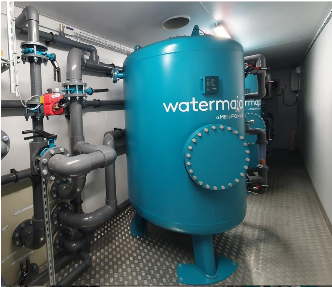
Figur 20, Installerat filtersystem i filtercontainer.
