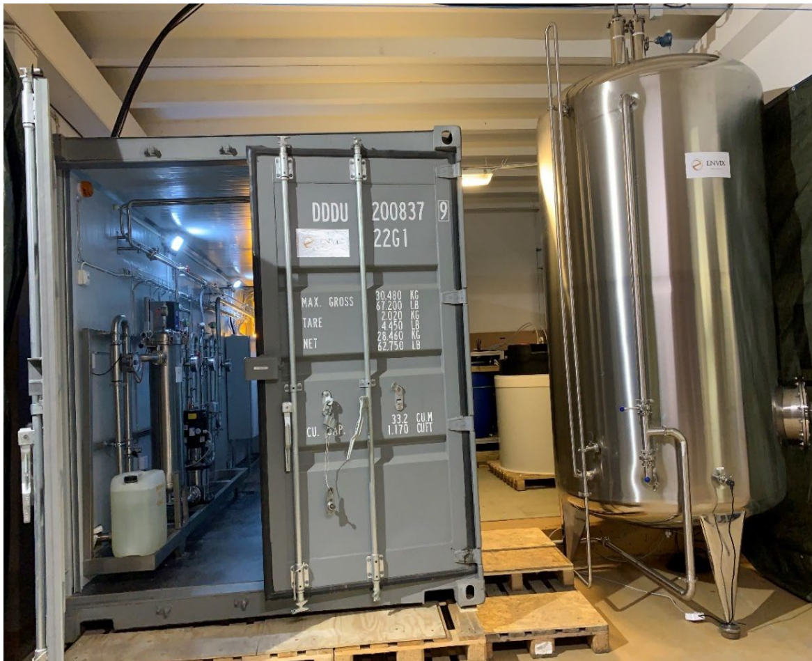
Figure 3. Photo of E-peroxone pilot system at Strömsund sewage treatment plant.
